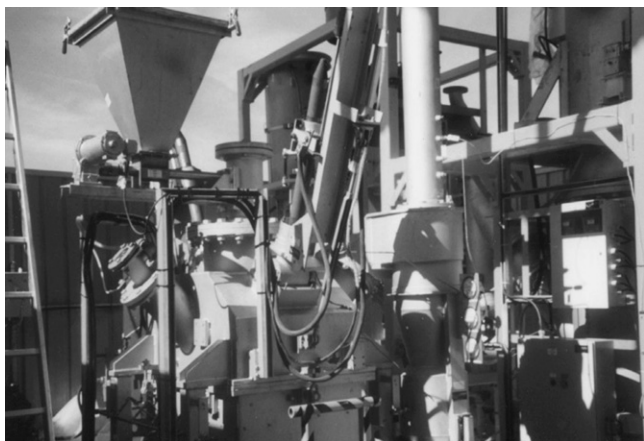
Fig. 1. Furnace and its related equipment.
